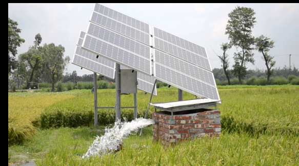
Solar Powered Irrigation Pumps
