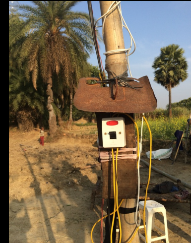
Electric Pump Sets
